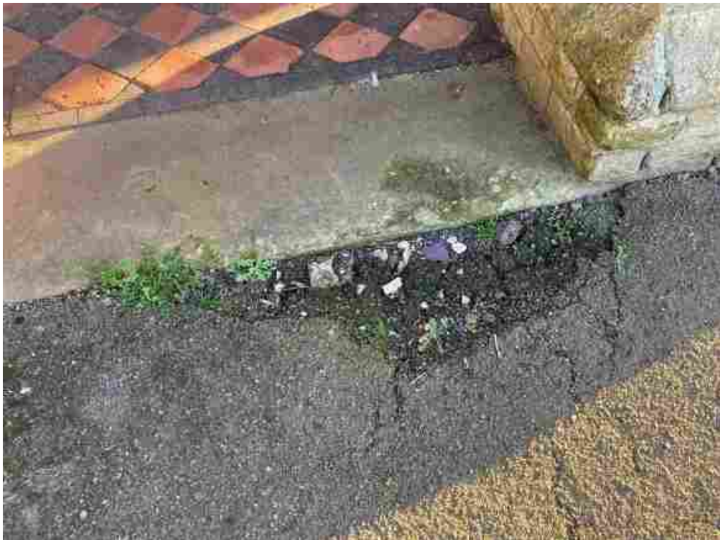
Failed section of asphalt.
