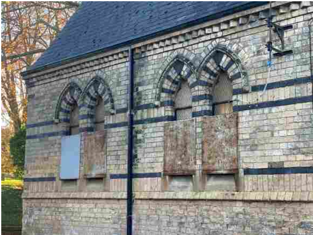
Security panels should be removed.
