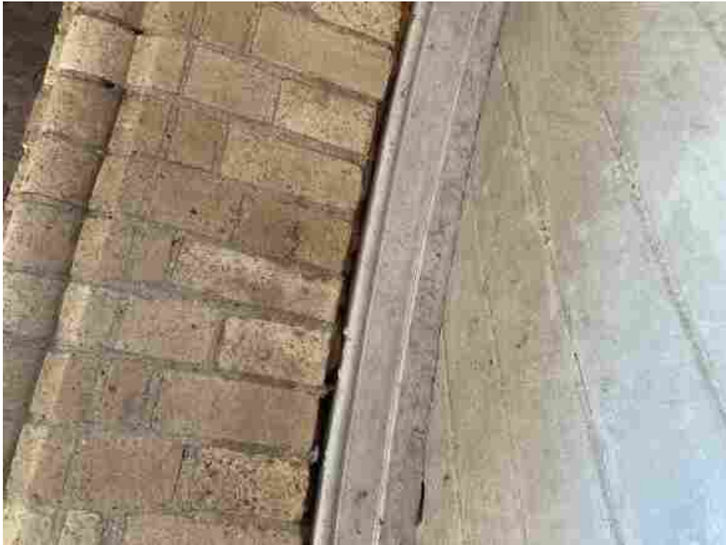
Missing mortar to doors/brickwork junction.
