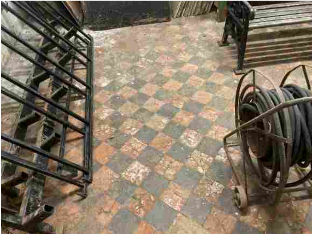
Heavy decay and damage to quarry tiles.
