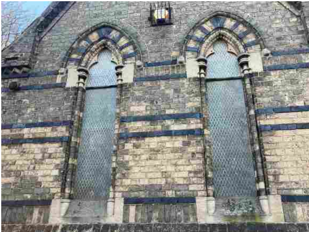
Fibreglass windows should be replaced.
