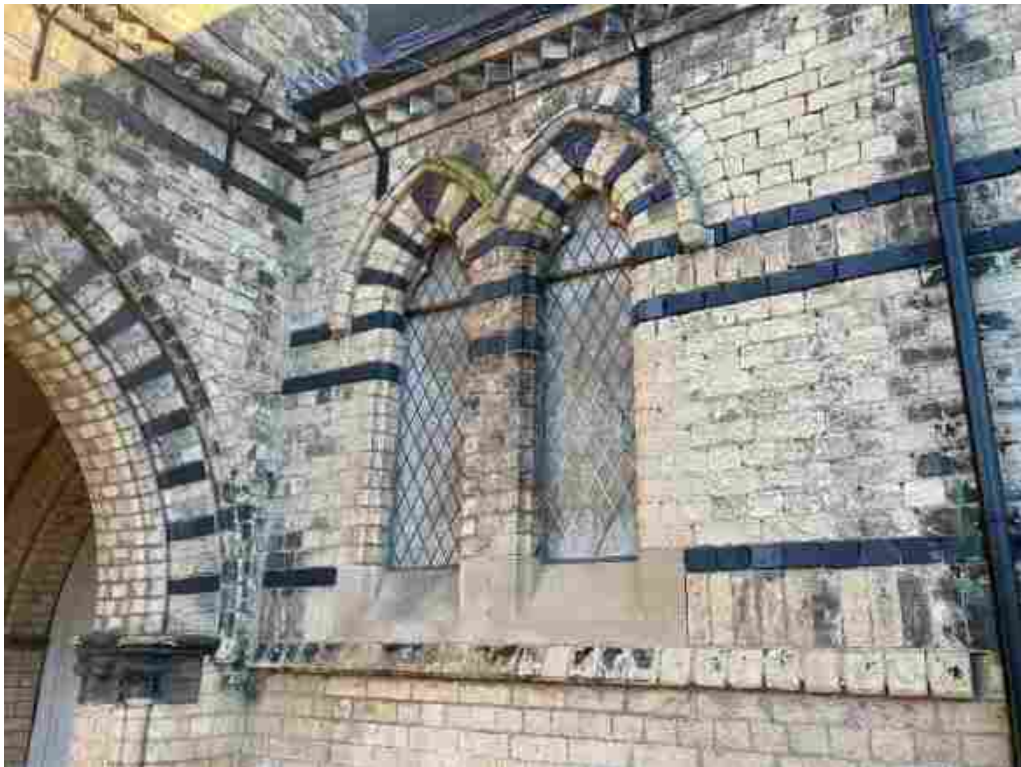
Fibreglass windows should be replaced.
