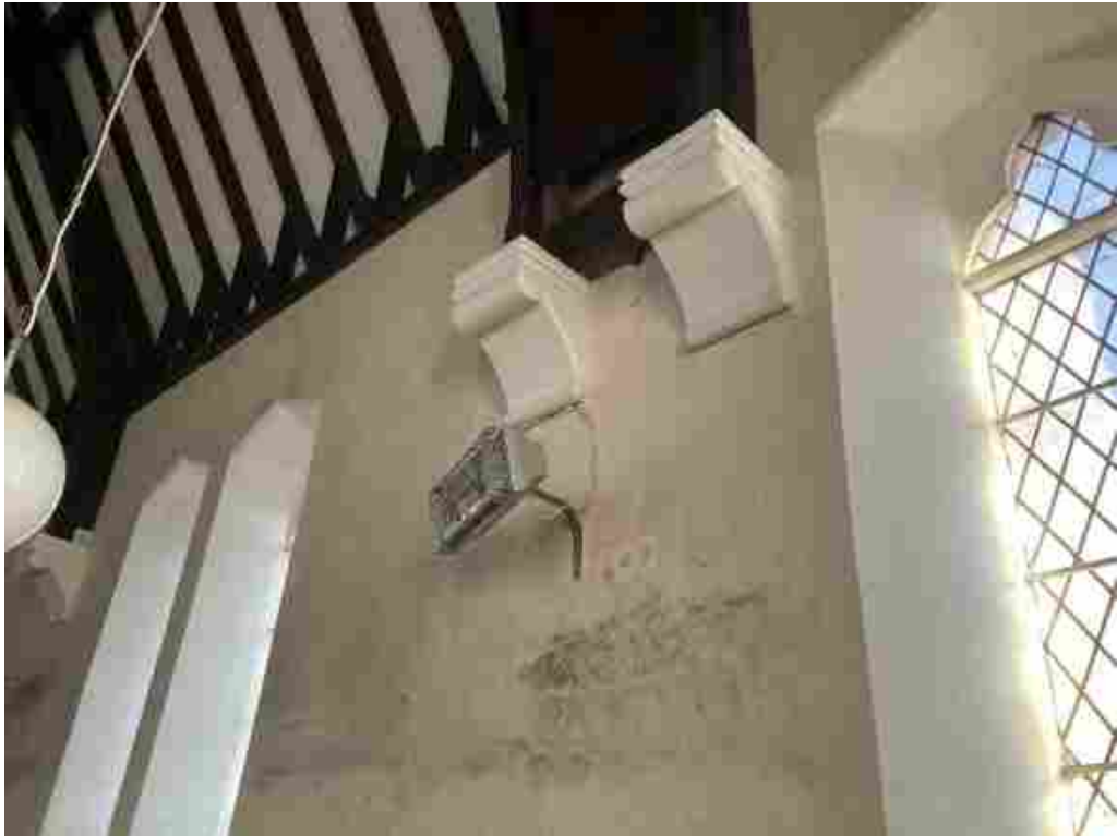
Infrared heating system to be replaced.
