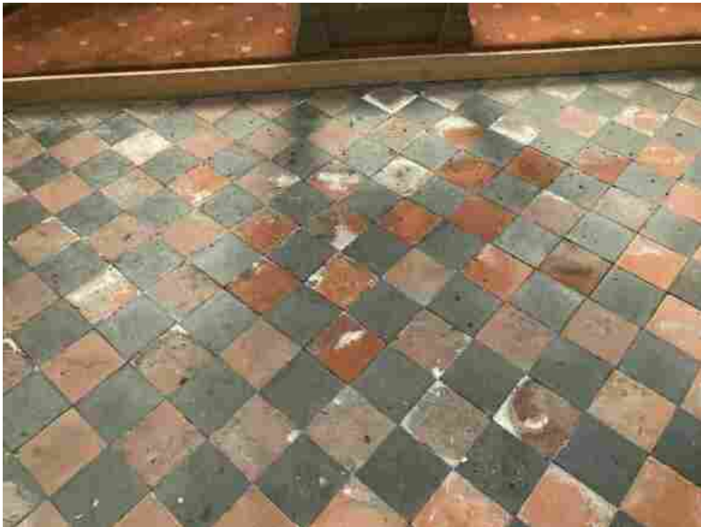
Decay to Chapel quarry tiles.
