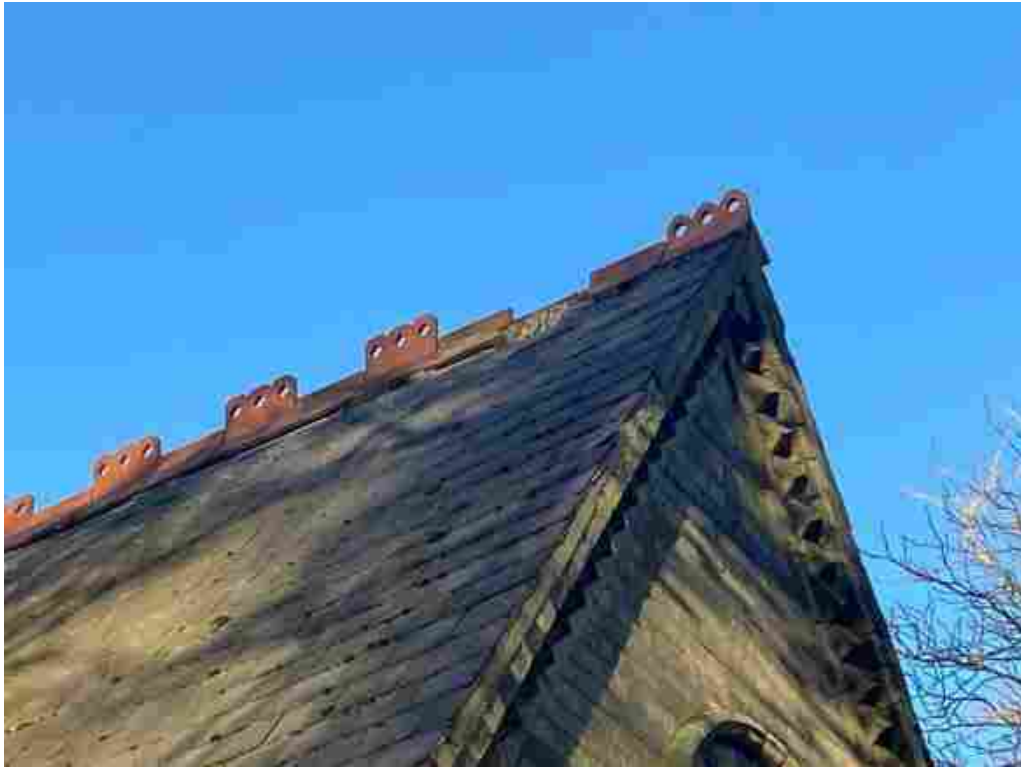
Missing decorative ridge tiles.
