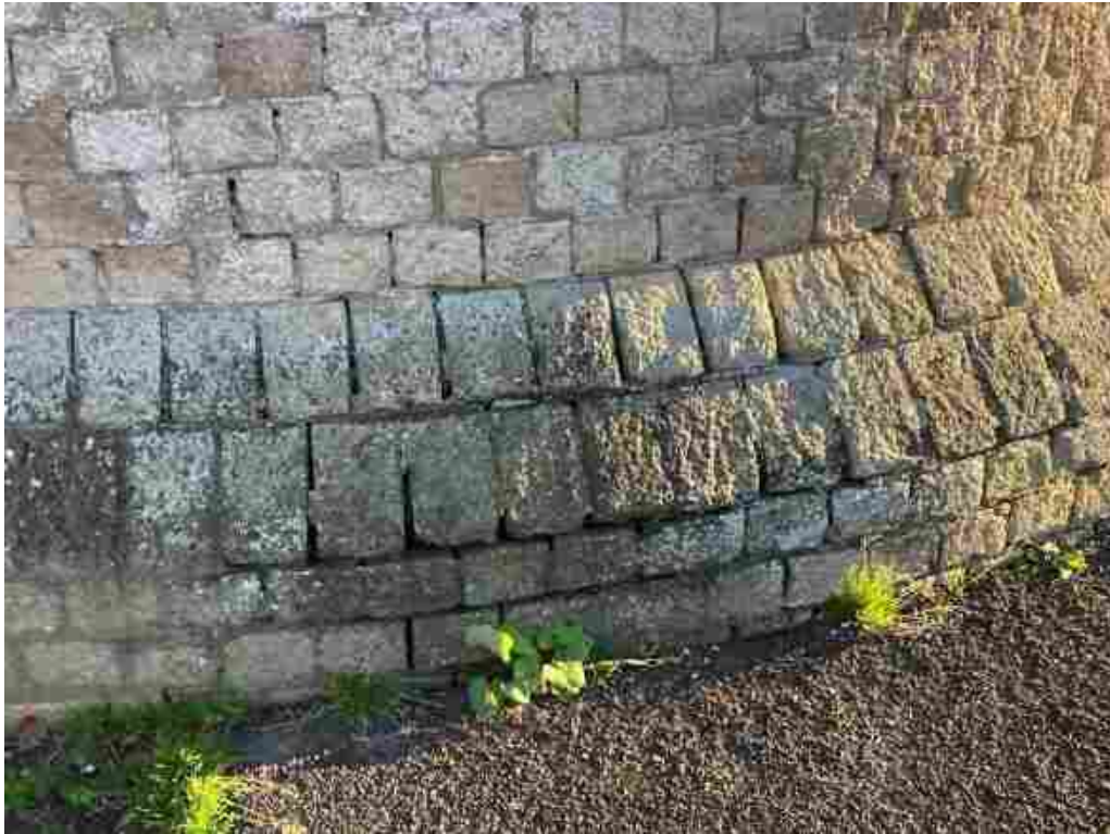
Open mortar joints to plinth.
