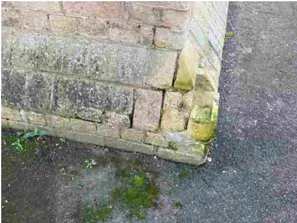
Section of missing brickwork to be rebuilt.
