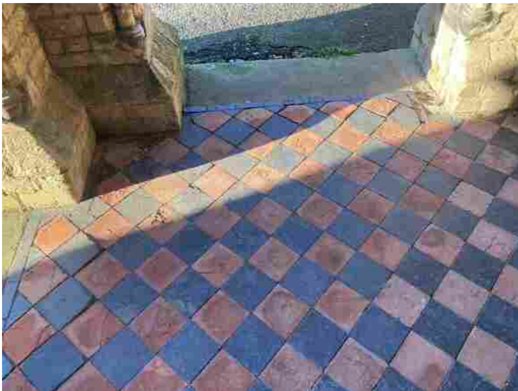
Decay and unevenness to quarry tiles.
