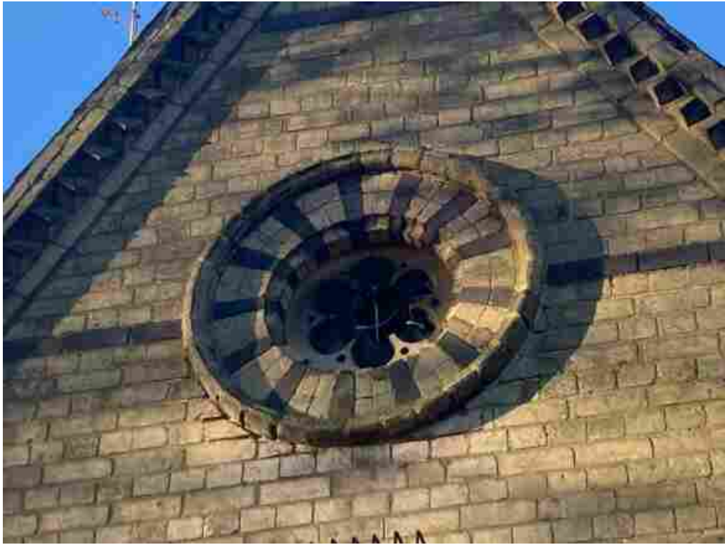
Broken round window on East elevation.
