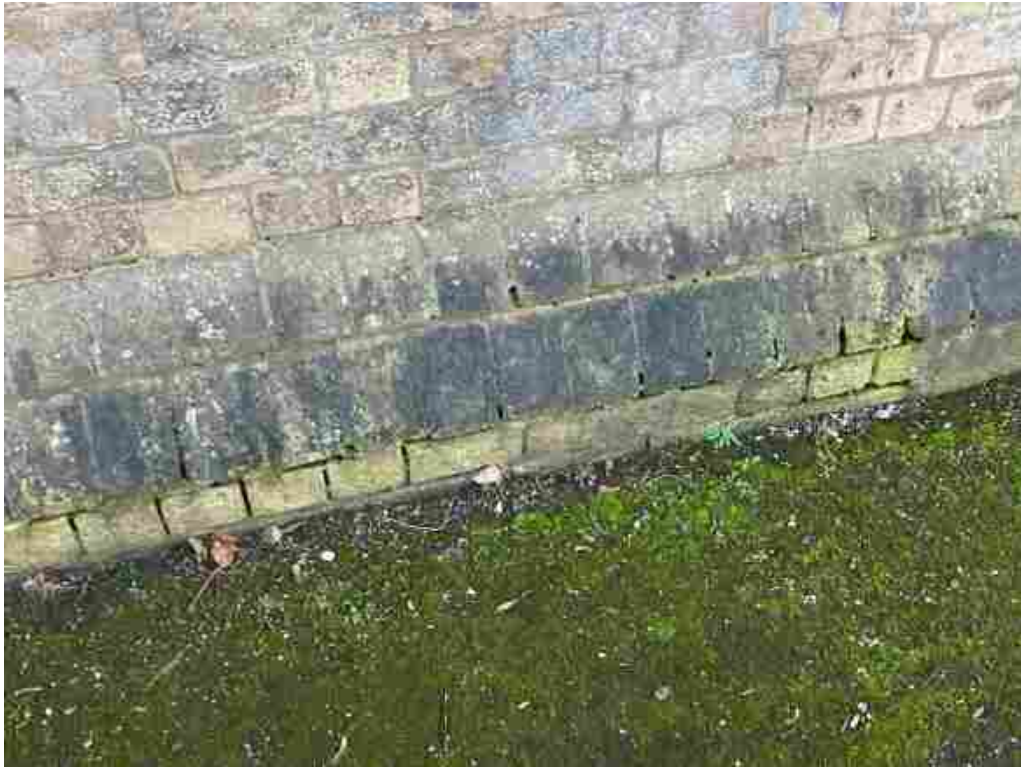
Open joints to plinth.
