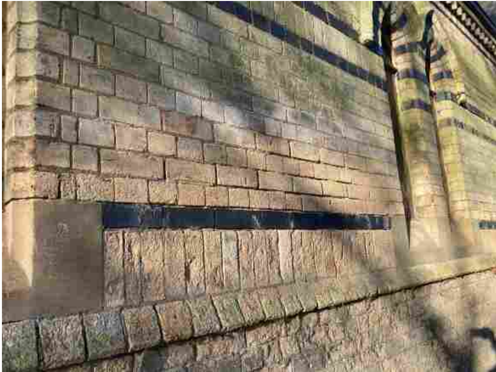
Open jointing to brickwork on East elevation.
