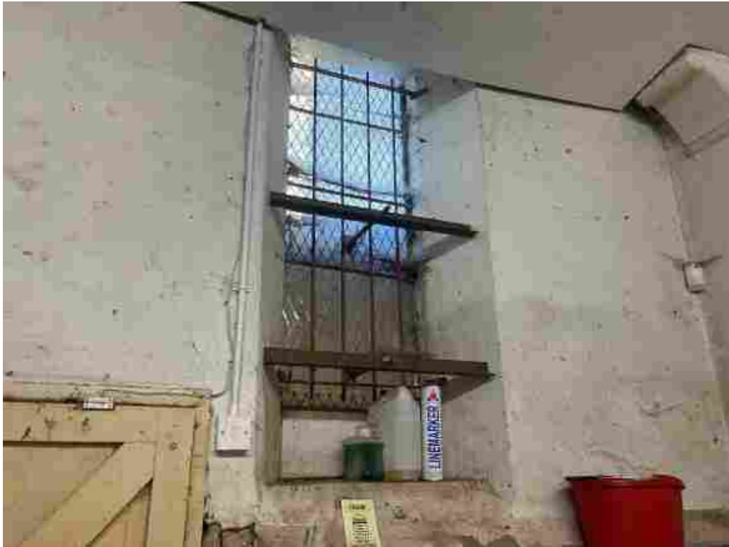
Fibreglass windows should be replaced.
