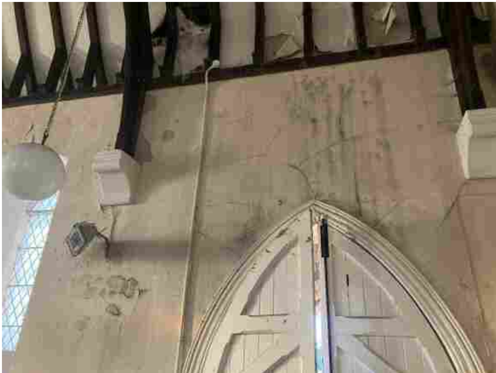
Widespread mould growth and failing paintwork.
