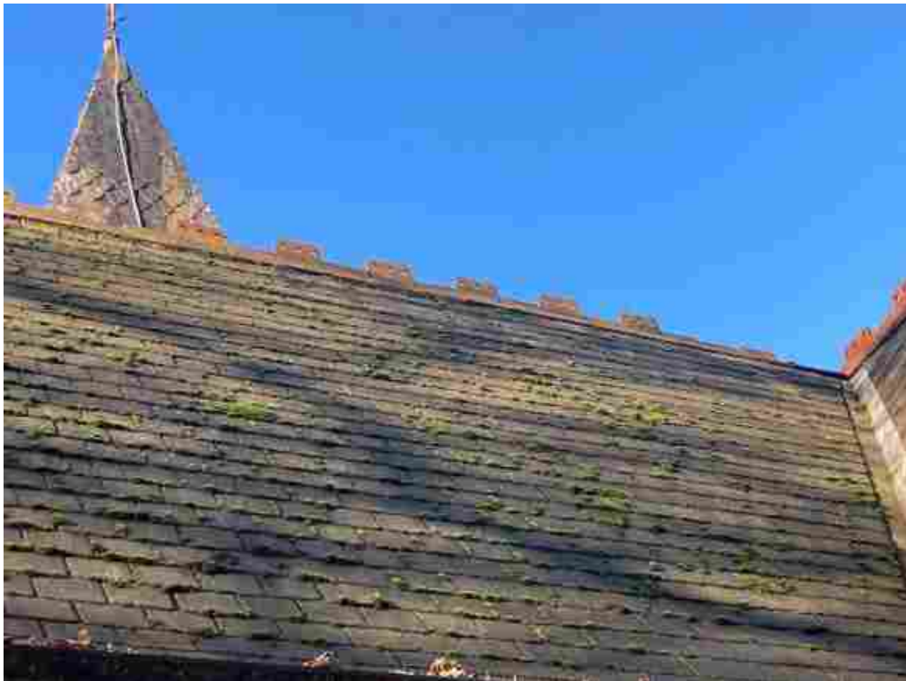
Moss buildup to Chapel should be cleared.
