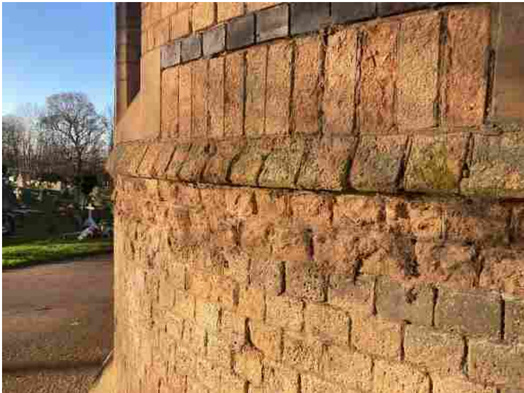
Area of brickwork replacements and pointing required.
