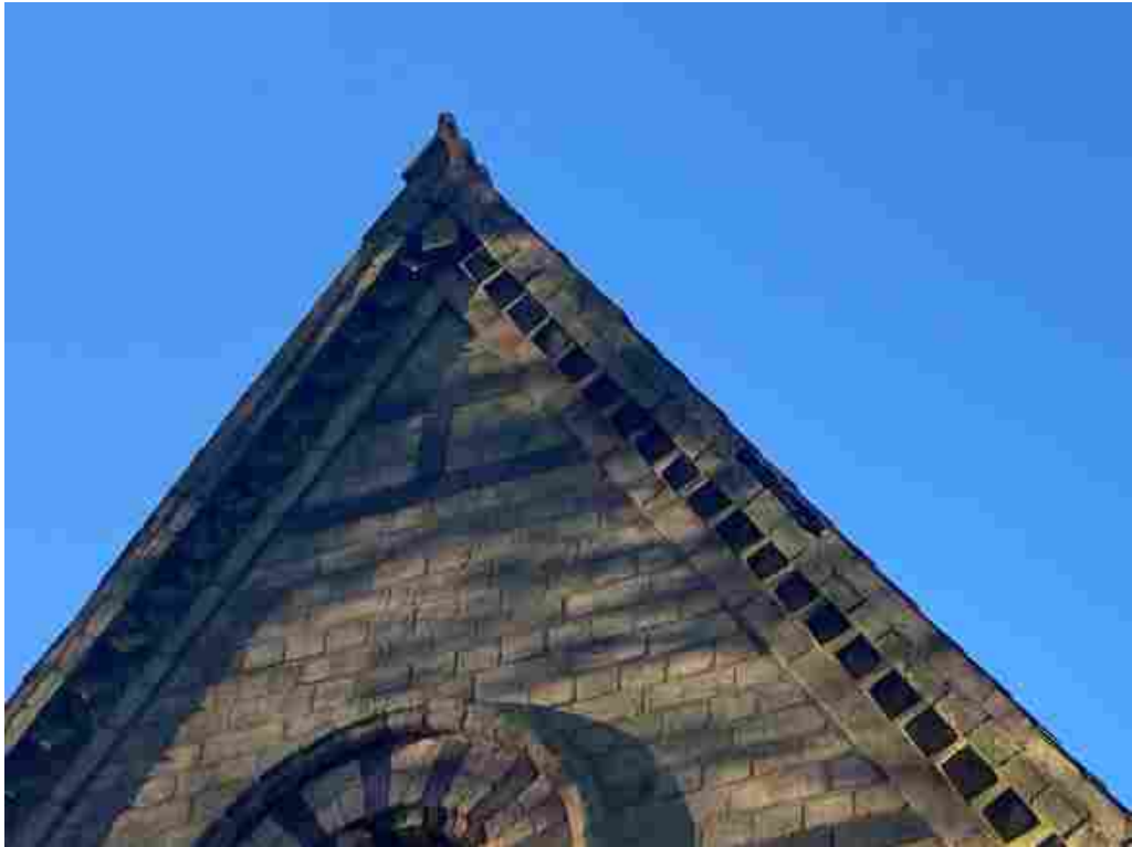
Missing or cracked verge pointing.
