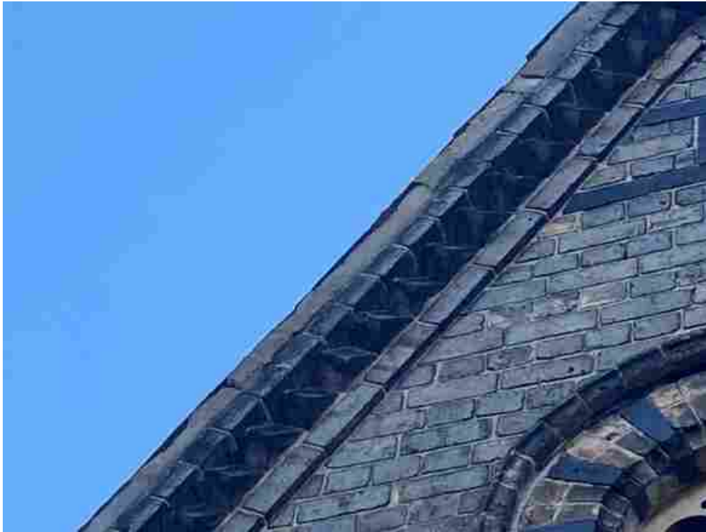
Missing verge pointing.
