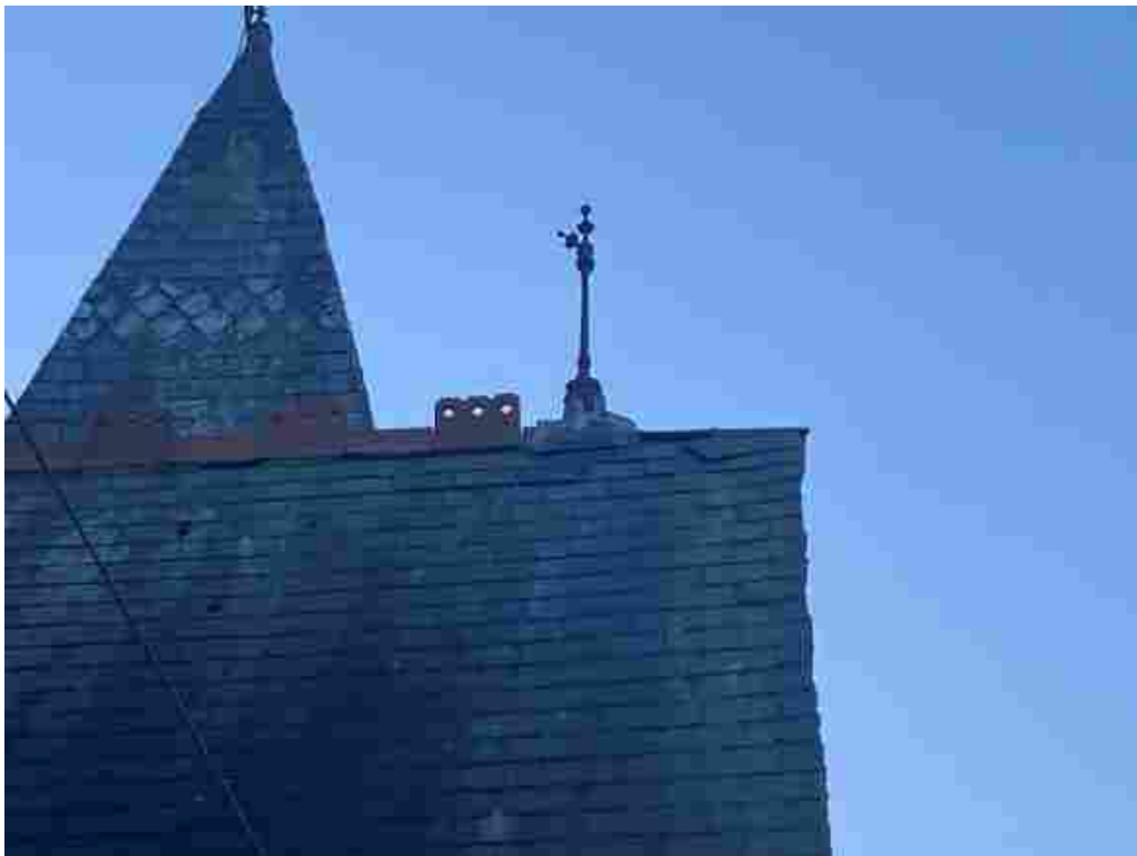
Loose slate and missing decorative ridge tiles.
