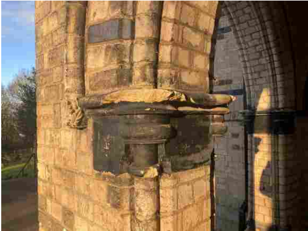
Stone decay to column capital.
