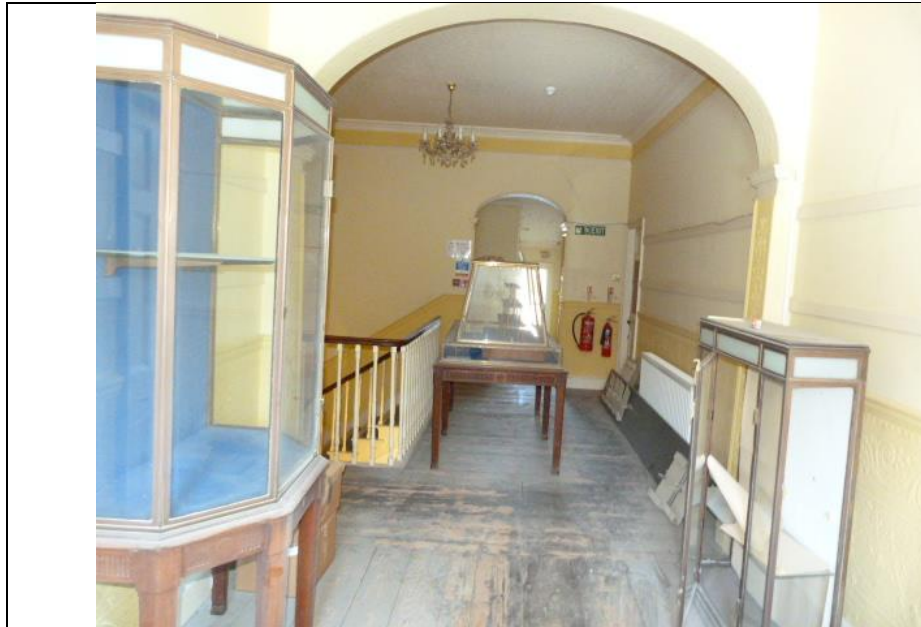
Item 36 Combustibles on the first-floor landing Priority: Medium
