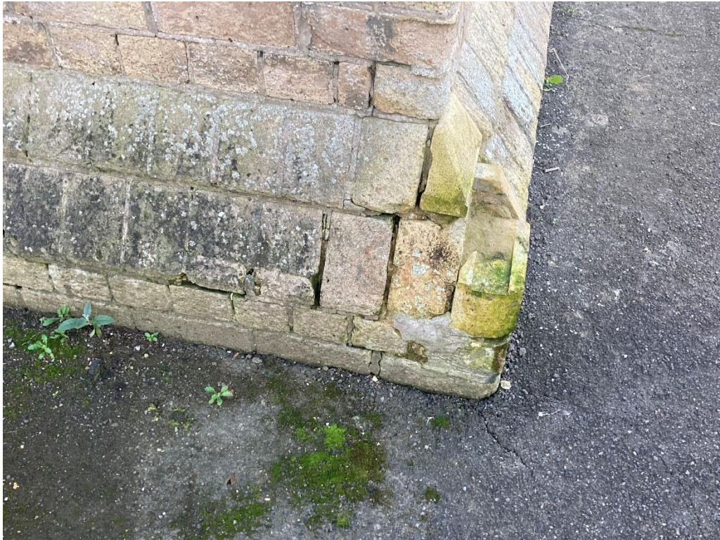
Section of missing brickwork to be rebuilt.
