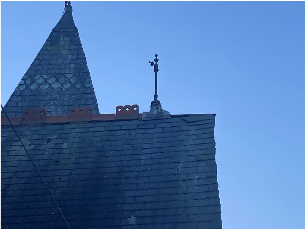
Loose slate and missing decorative ridge tiles.
