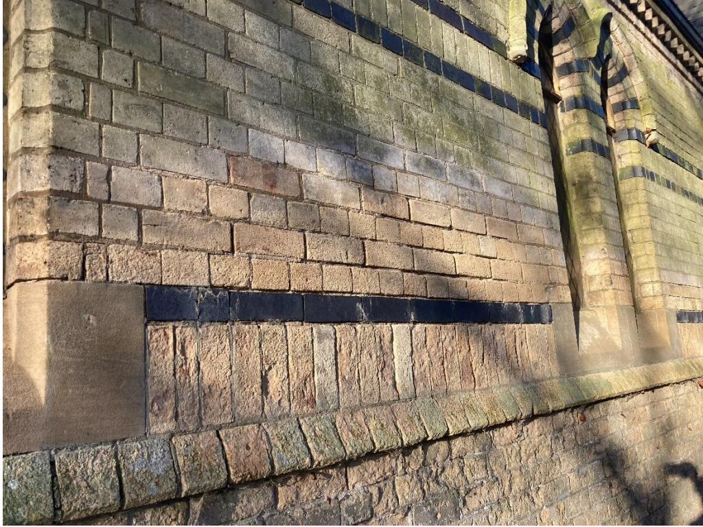
Open jointing to brickwork on East elevation.
