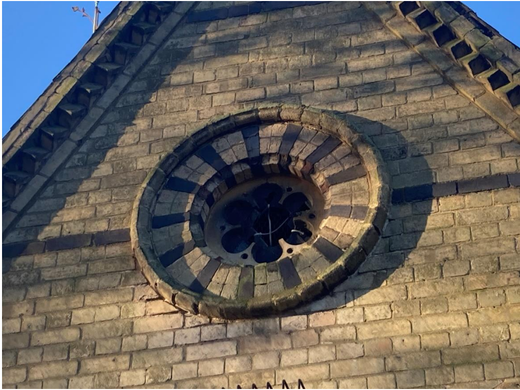
Broken round window on East elevation.
