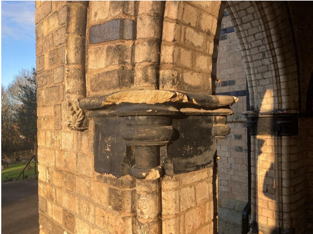
Stone decay to column capital.
