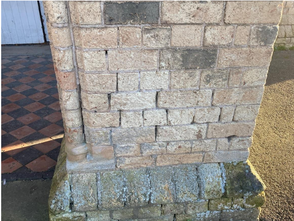
Open joints in cementitious mortar to Tower arch.
