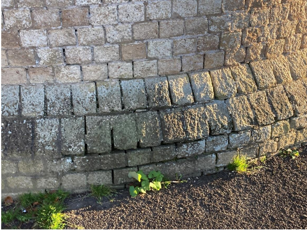
Open mortar joints to plinth.
