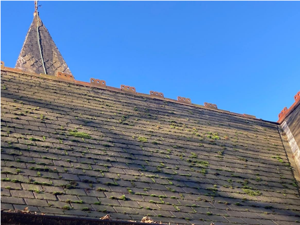
Moss buildup to Chapel should be cleared.
