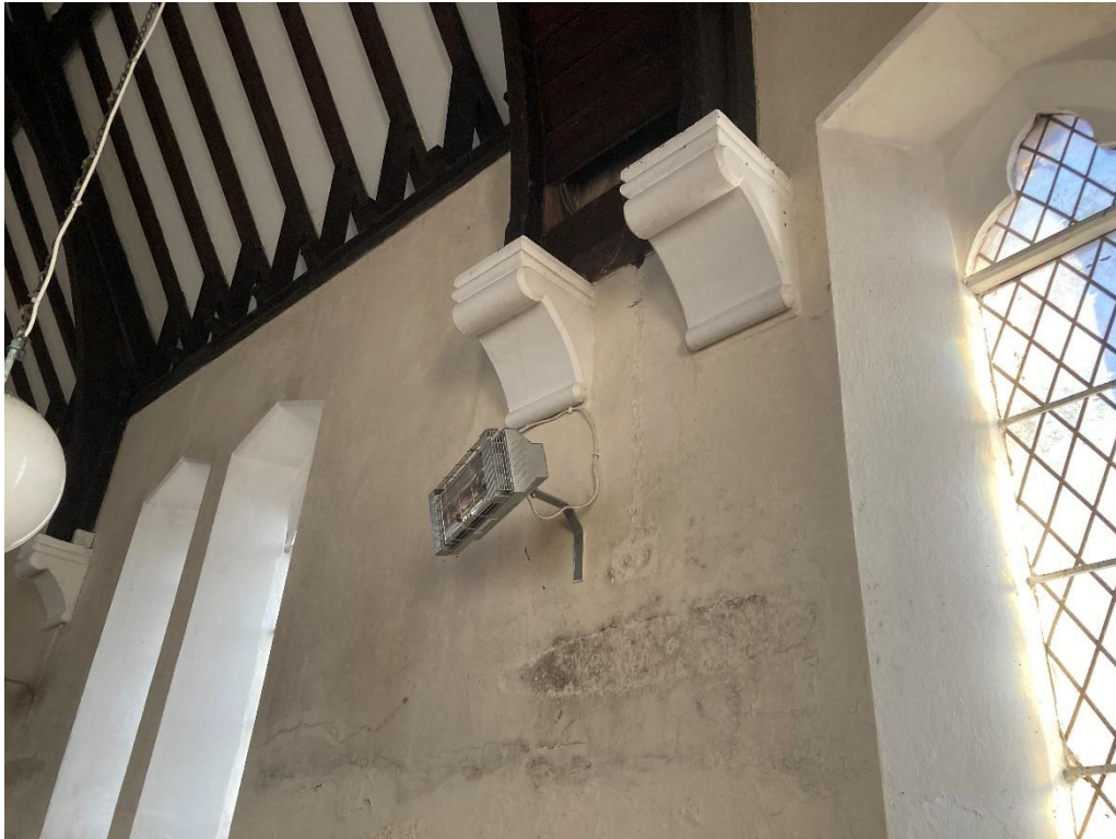
Infrared heating system to be replaced.
