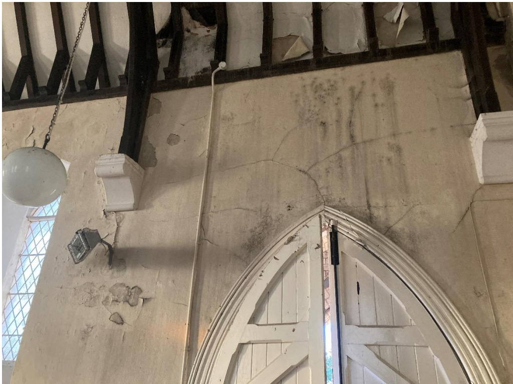
Widespread mould growth and failing paintwork.
