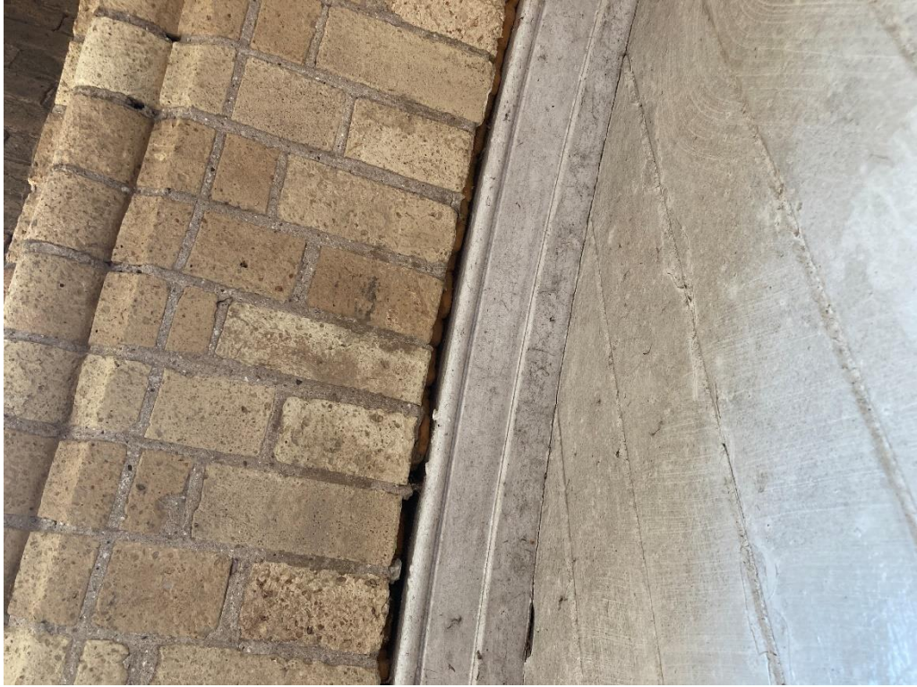
Missing mortar to doors/brickwork junction.
