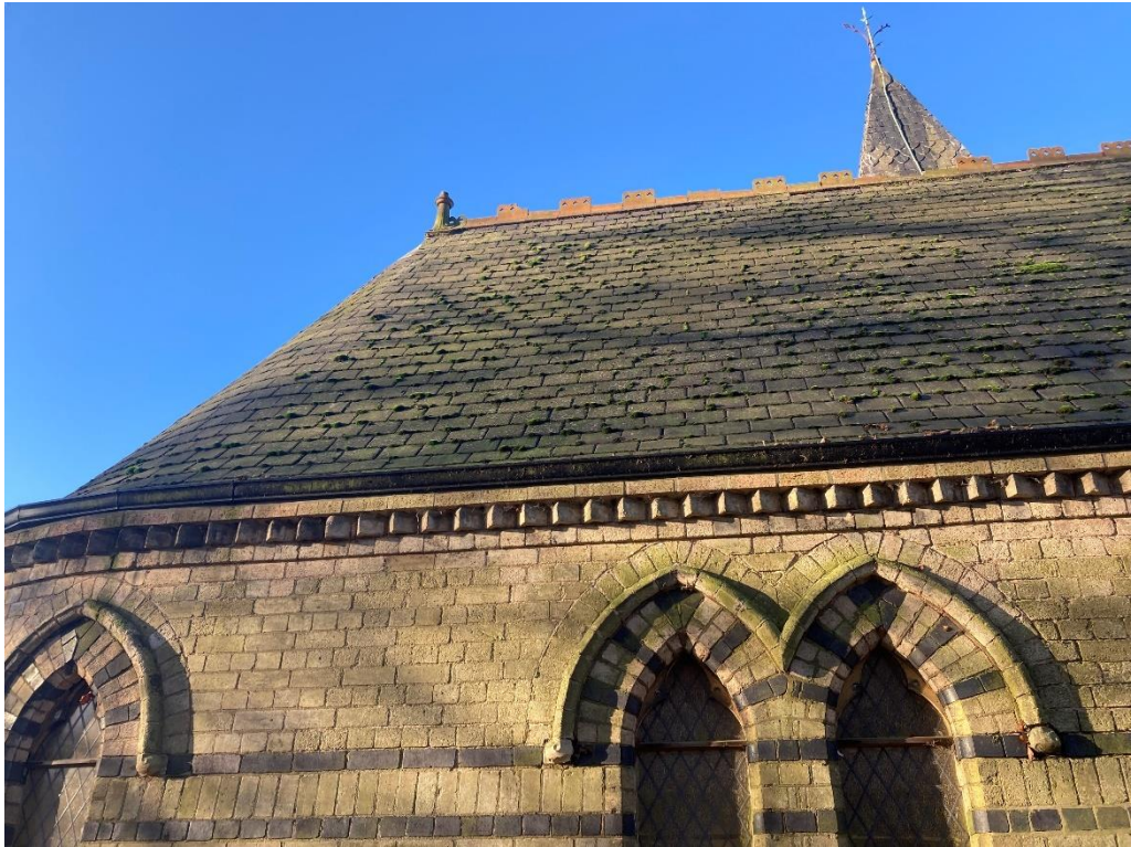
Slating generally appears in satisfactory condition, barring missing ridge tiles and pointing.
