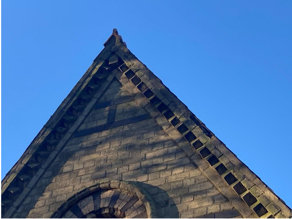
Missing or cracked verge pointing.
