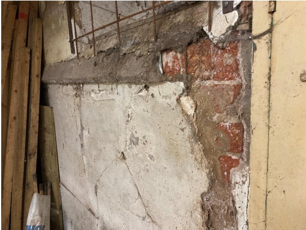
Cementitious render has also been used in this area, which should be removed.
