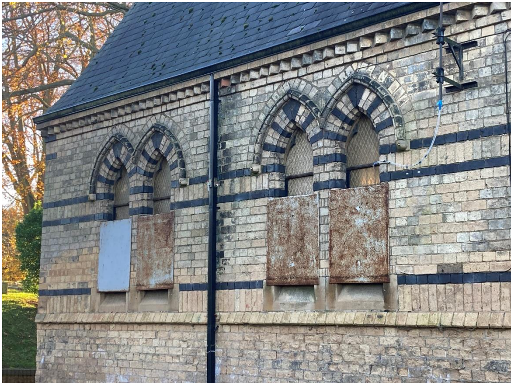
Security panels should be removed.
