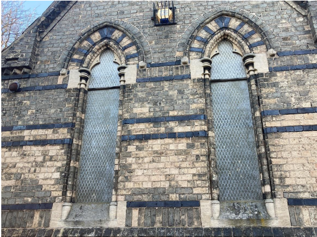
Fibreglass windows should be replaced.
