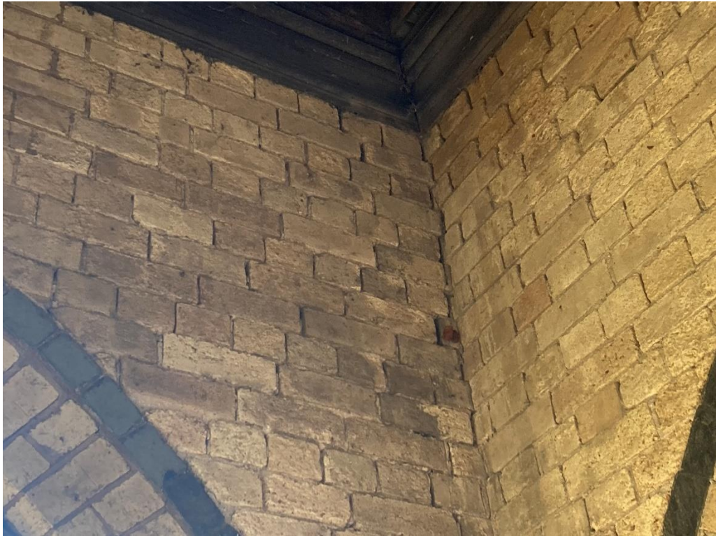
Recessed joints to the Tower base.
