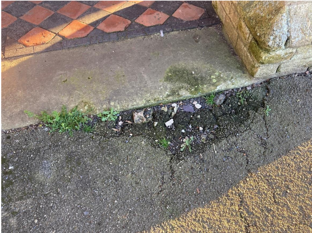
Failed section of asphalt.
