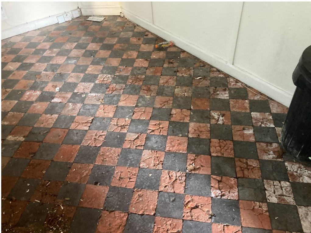
Severe decay and salting to quarry tiles in Meeting Room.
