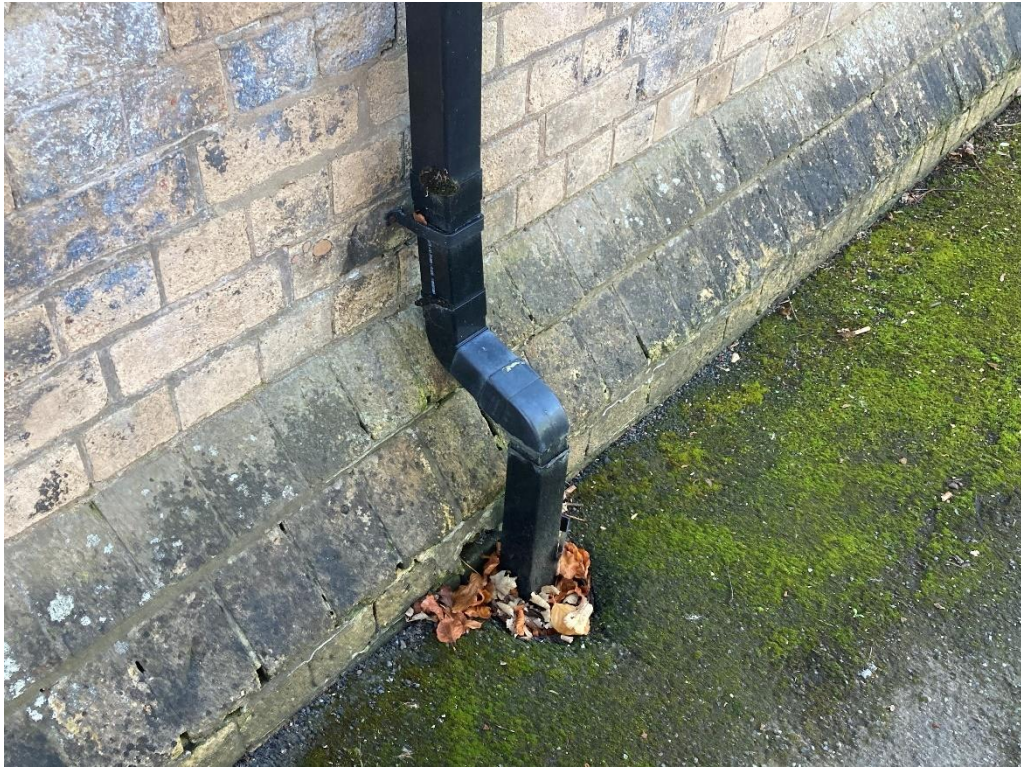
uPVC downpipes should be replaced with a more sympathetic material.
