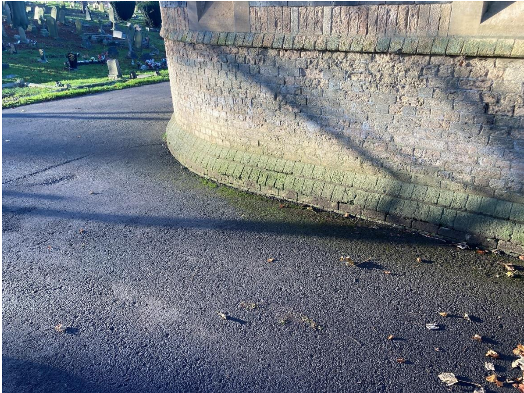
Asphalt has been installed up to the base of the wall, trapping moisture against the building.
