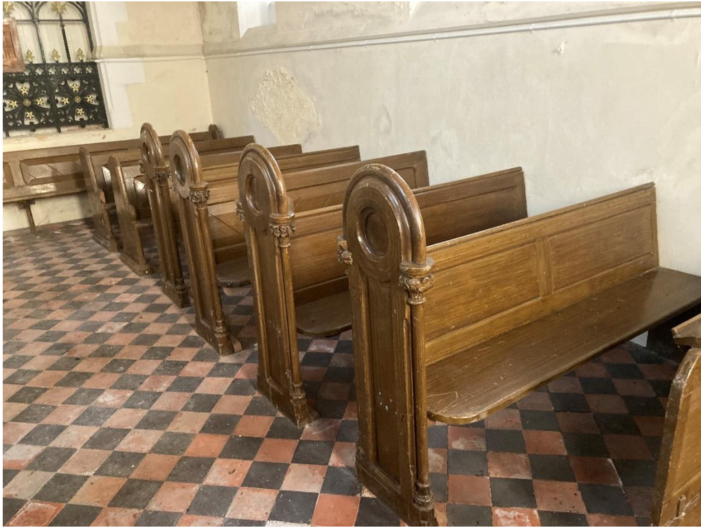
Some pews are loose. A more flexible seating option could be considered.
