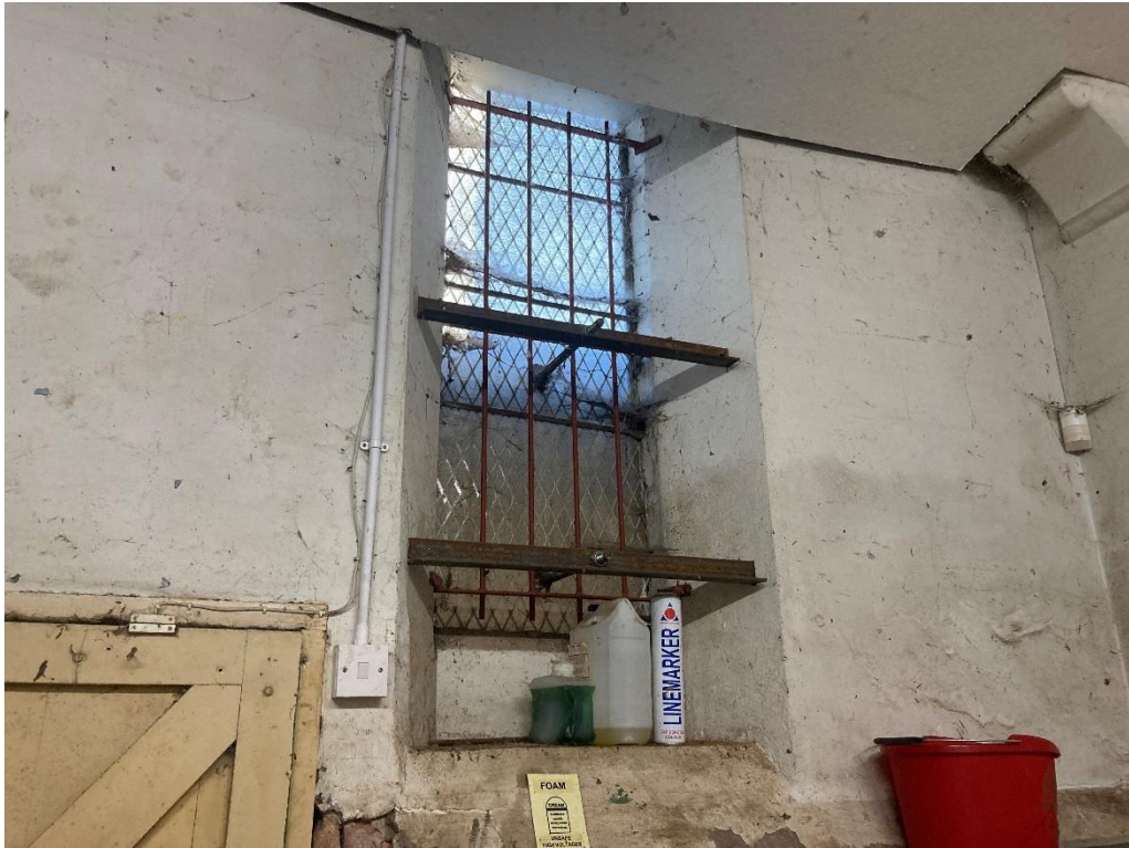
Fibreglass windows should be replaced.
