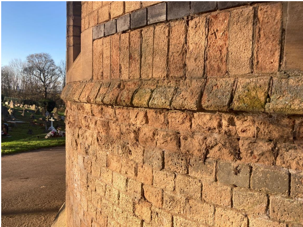
Area of brickwork replacements and pointing required.
