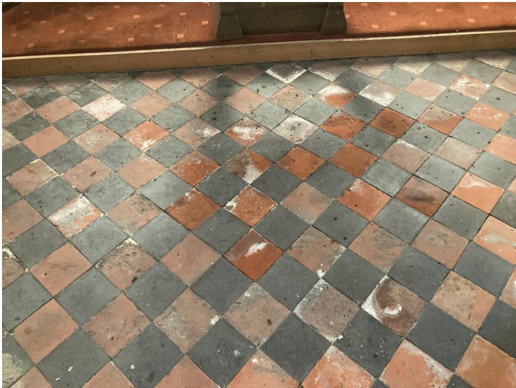
Decay to Chapel quarry tiles.
