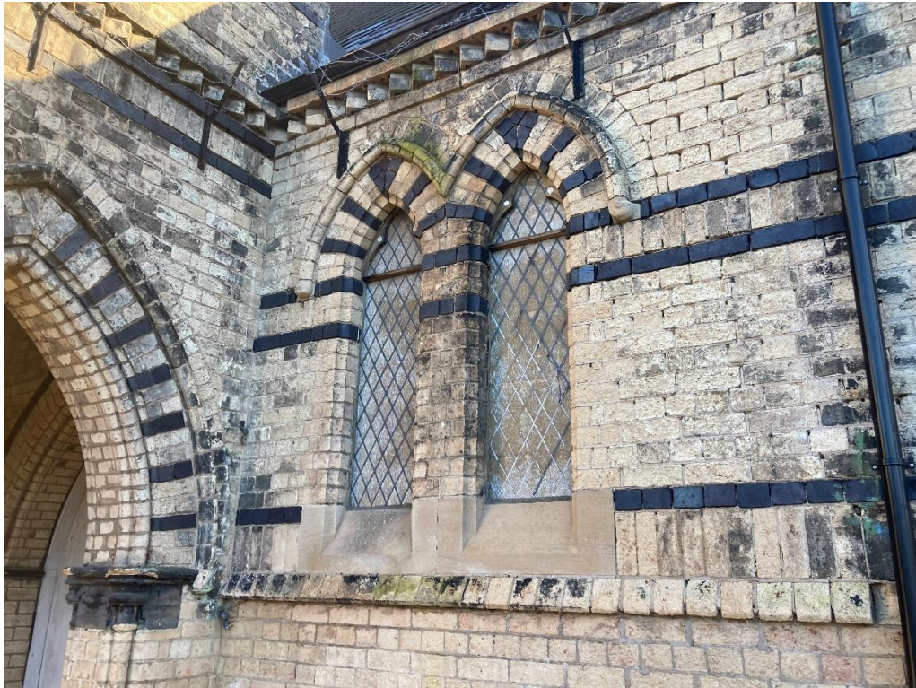
Fibreglass windows should be replaced.
