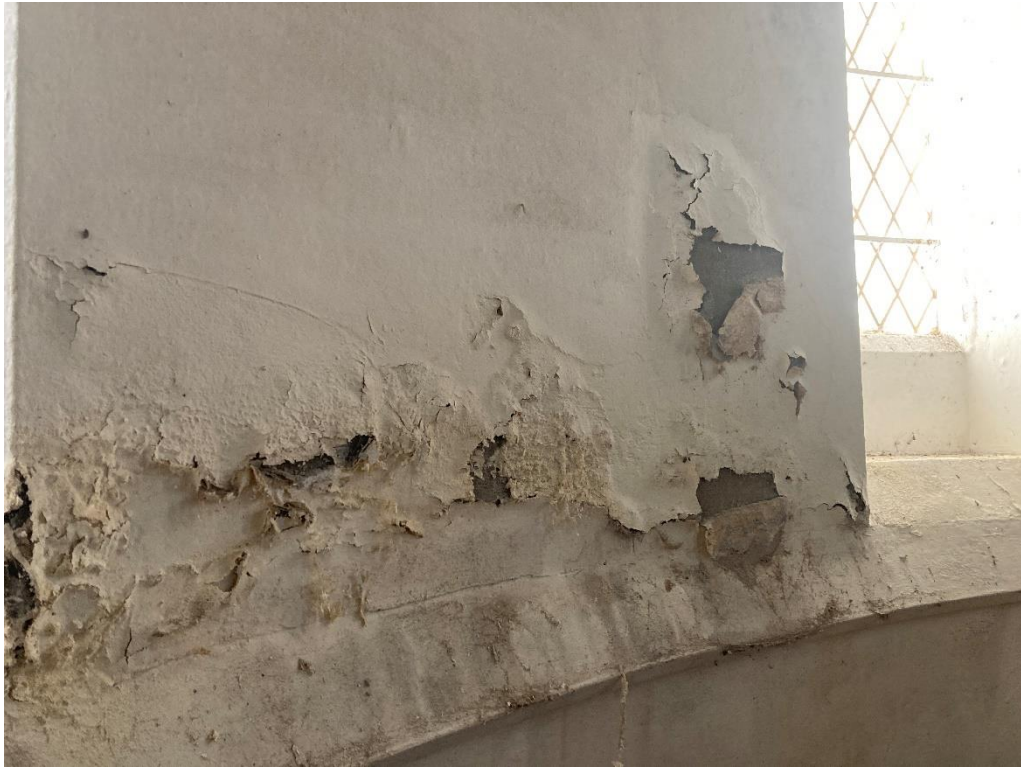
Cementitious render is causing widespread issues with damp.
