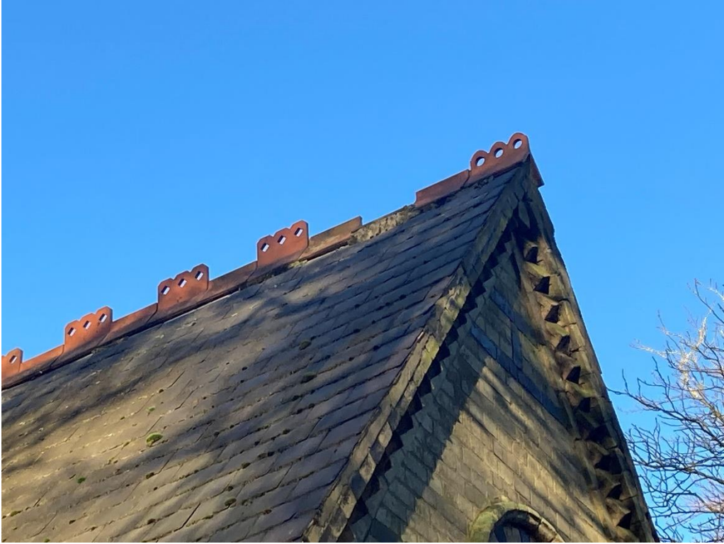
Missing decorative ridge tiles.
