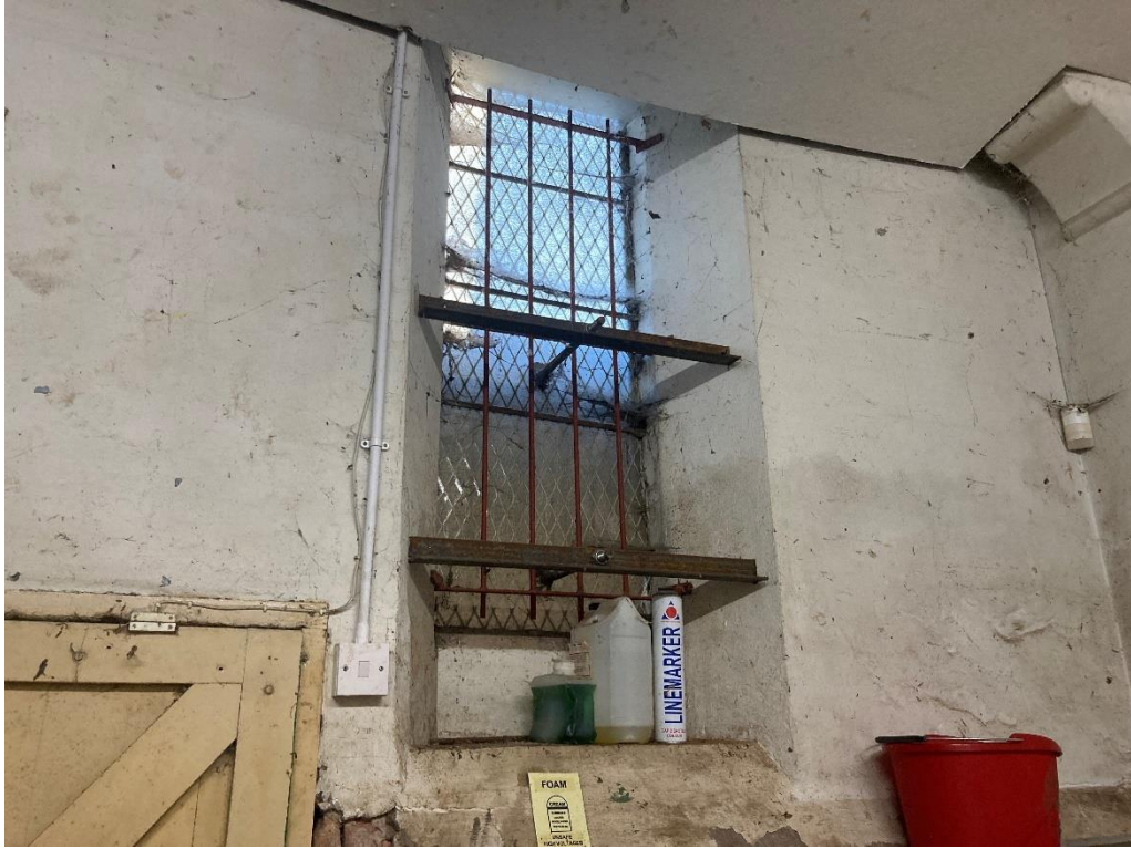
Fibreglass windows should be replaced.
