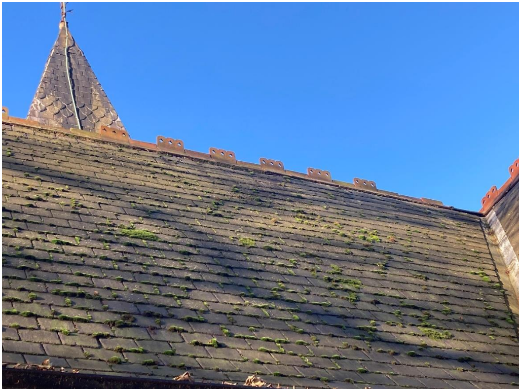
Moss buildup to Chapel should be cleared.
