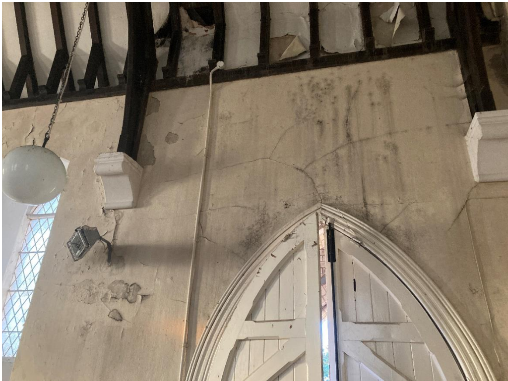
Widespread mould growth and failing paintwork.
