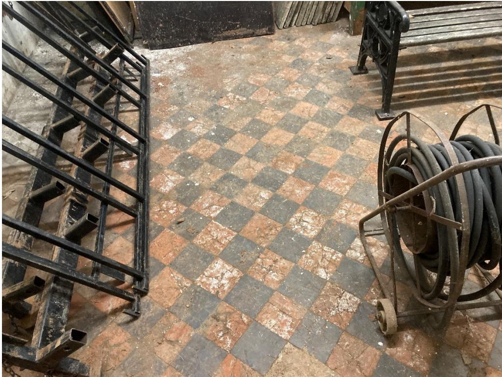
Heavy decay and damage to quarry tiles.
