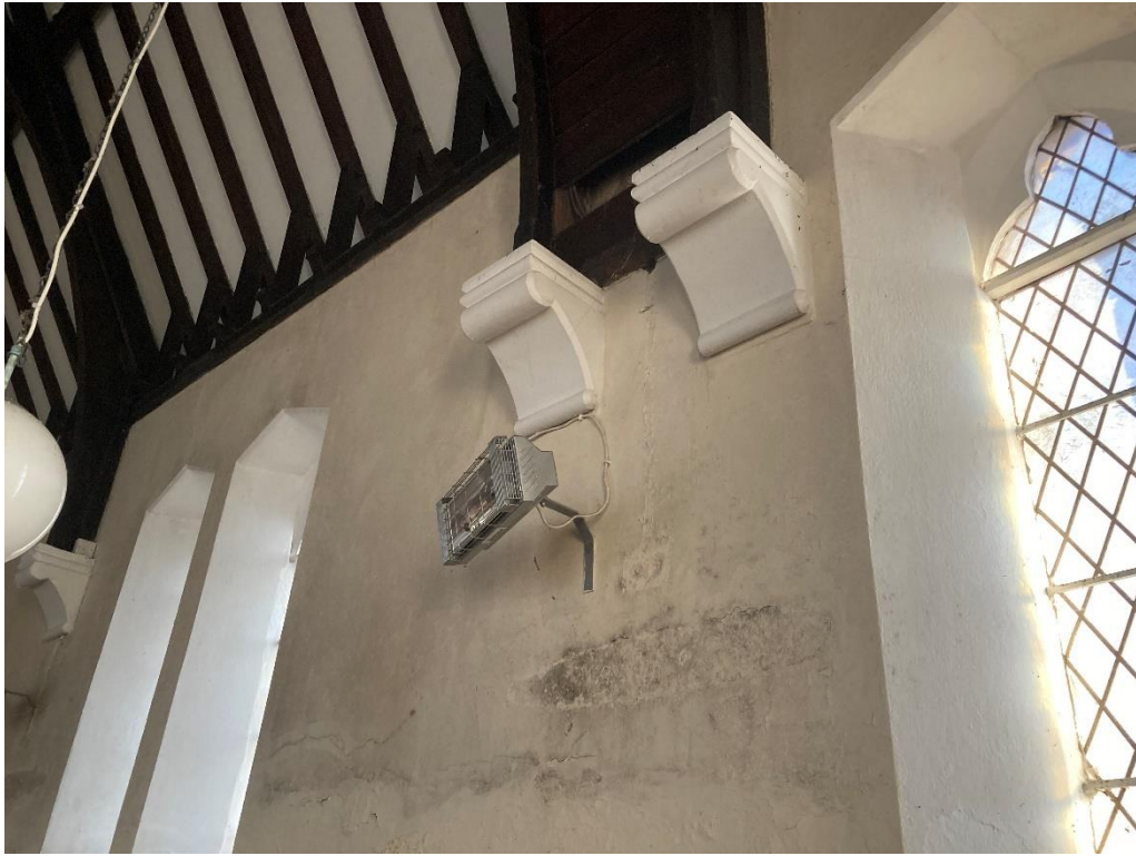
Infrared heating system to be replaced.
