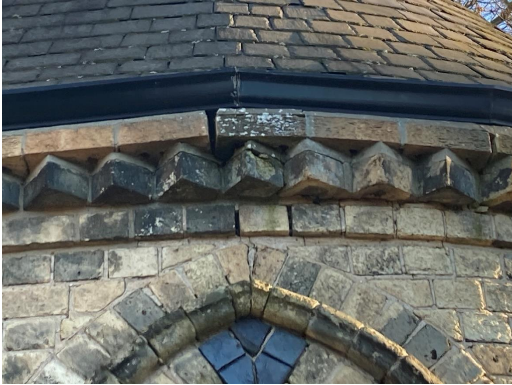
Crack to head of window extending up into the dogtooth brick cornice.
