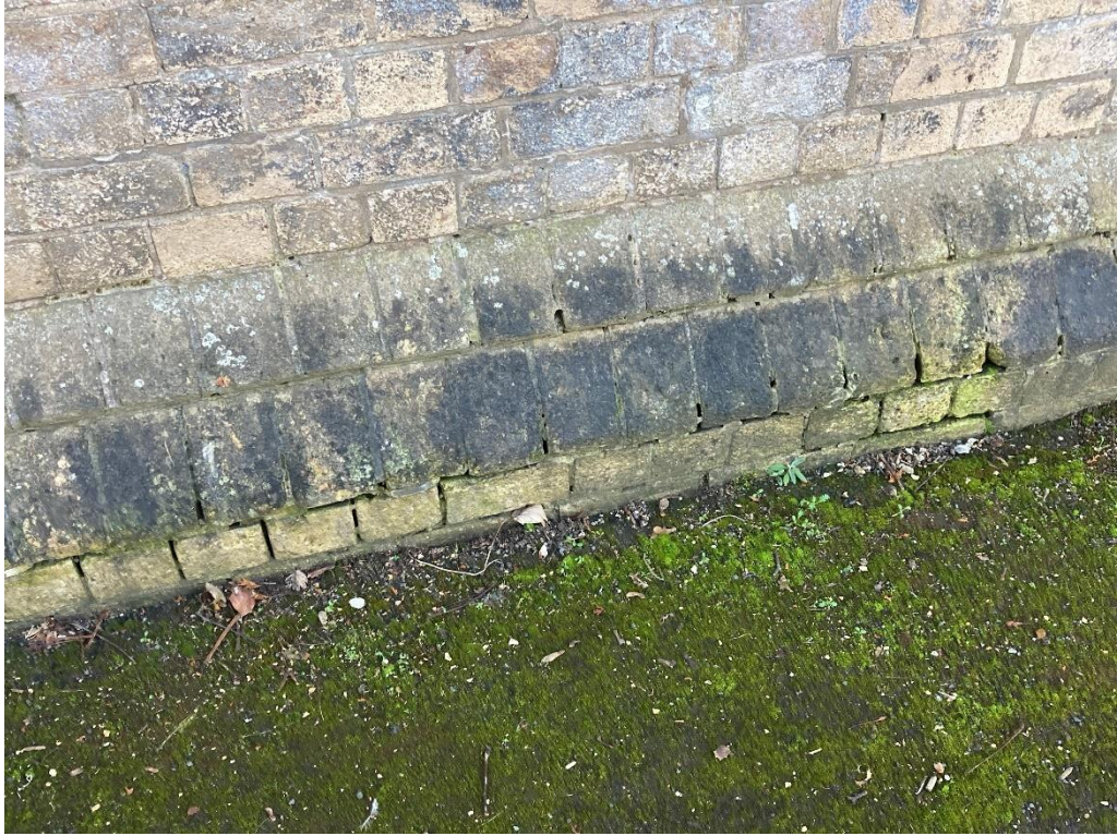
Open joints to plinth.
