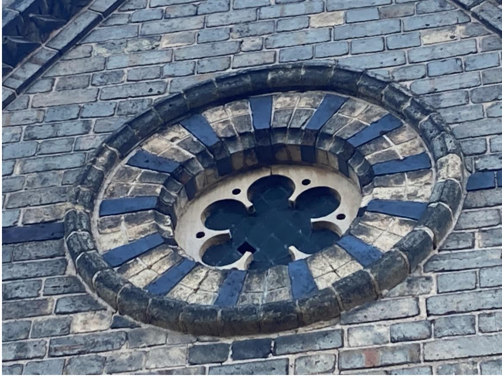
Missing quarry to round window on West elevation.
