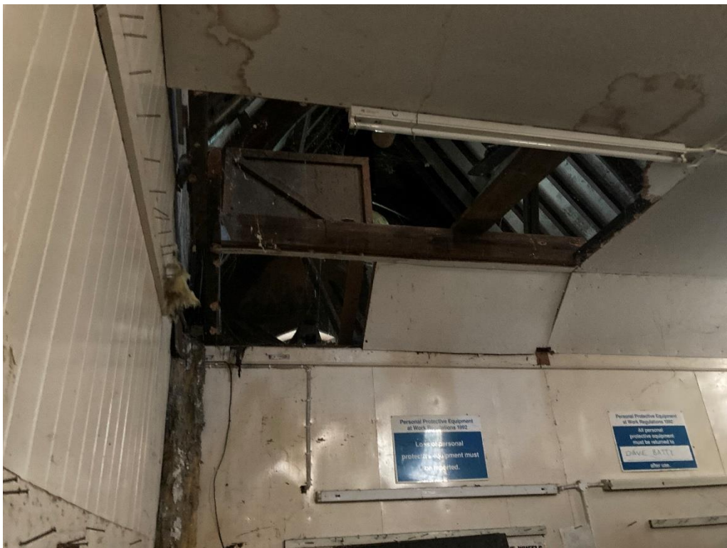
Further investigations should be undertaken when partitions removed or access provided.
