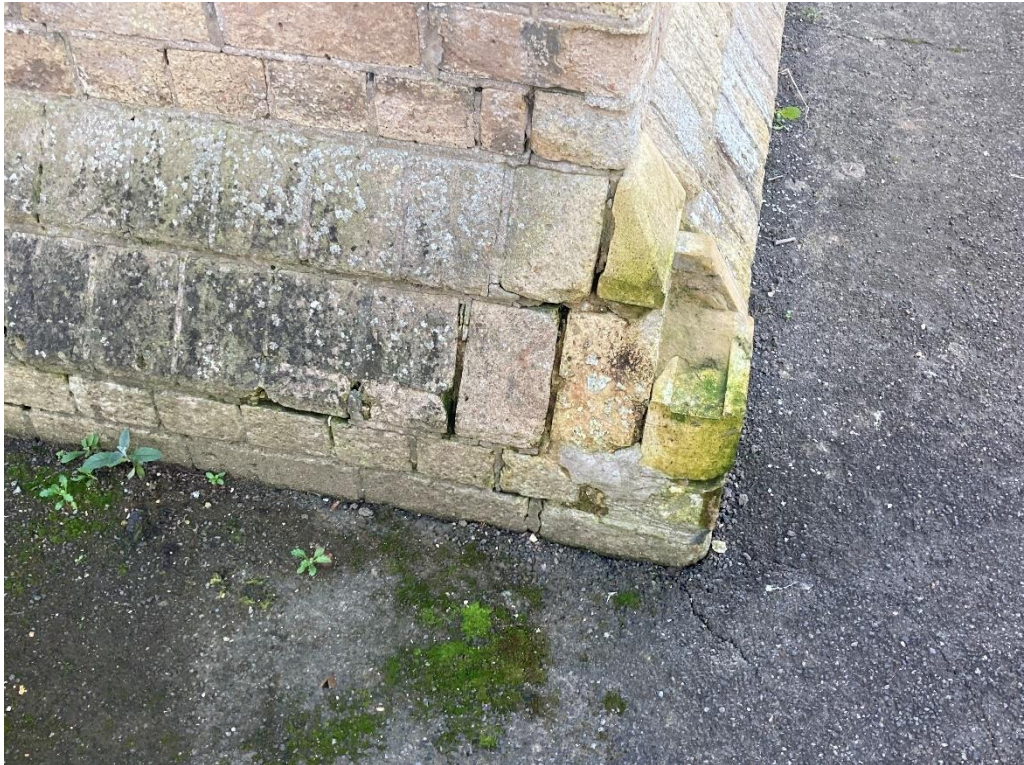
Section of missing brickwork to be rebuilt.
