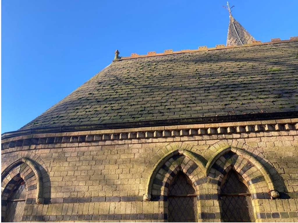
Slating generally appears in satisfactory condition, barring missing ridge tiles and pointing.
