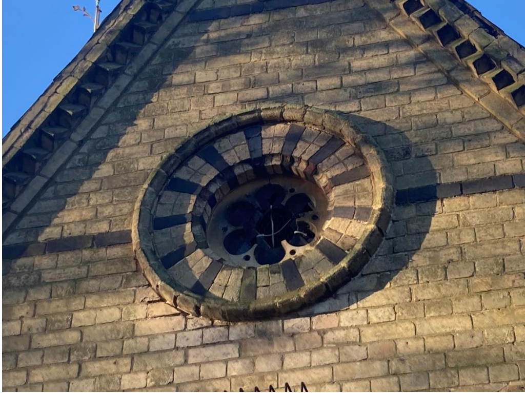
Broken round window on East elevation.
