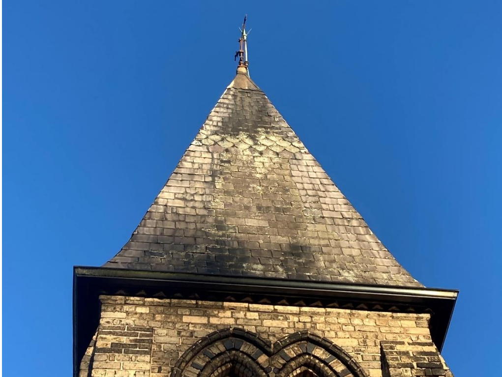
Slating appears to be in good condition, although gutters should be cleared.
