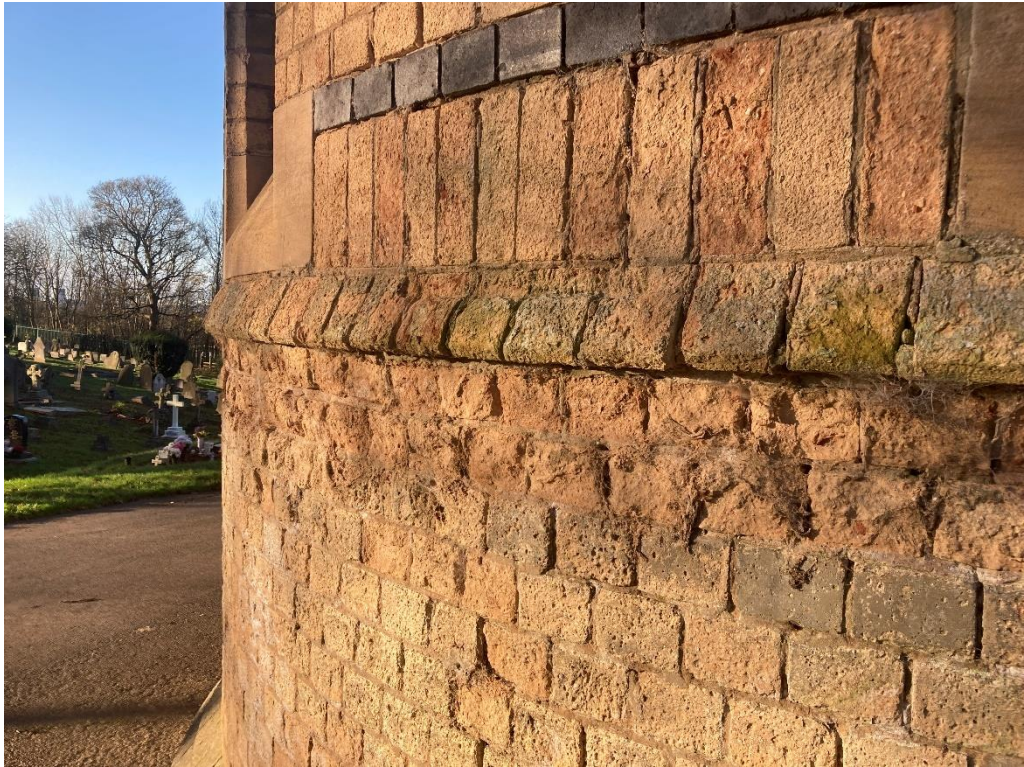
Area of brickwork replacements and pointing required.
