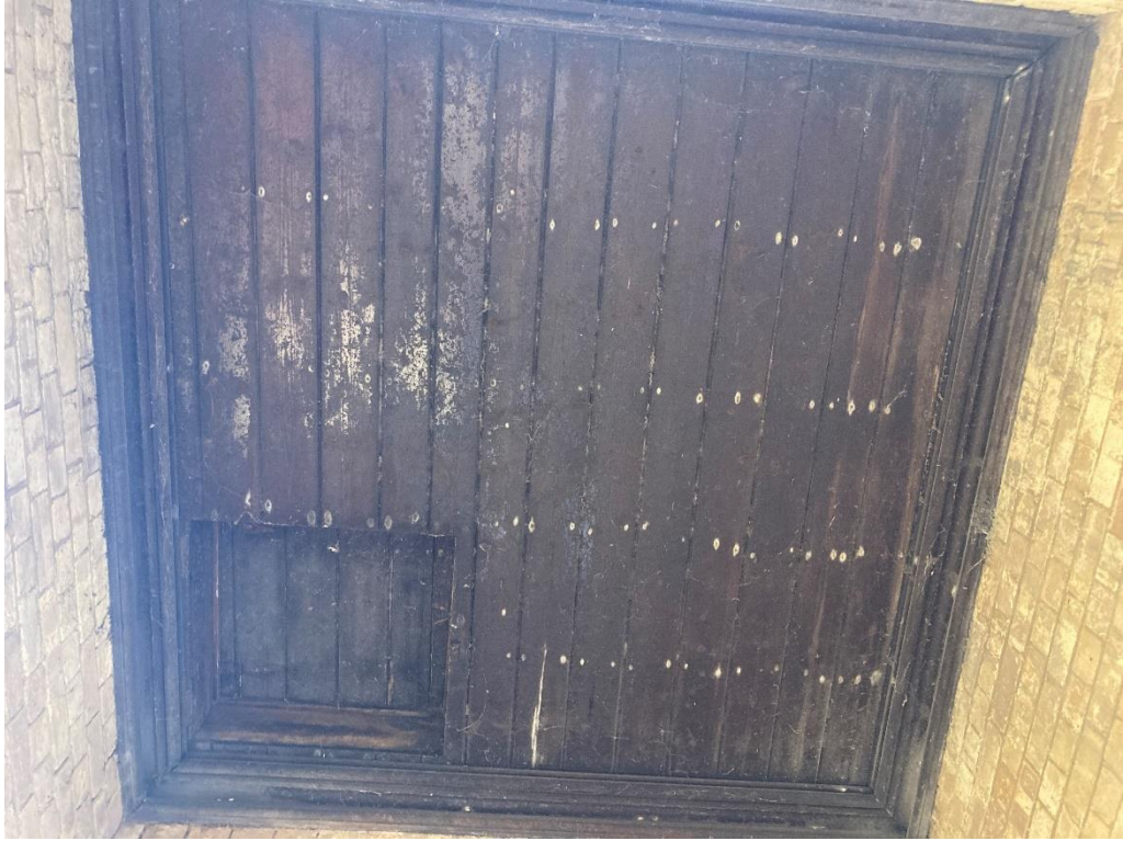
Further access should be given to investigate Belfry condition.
