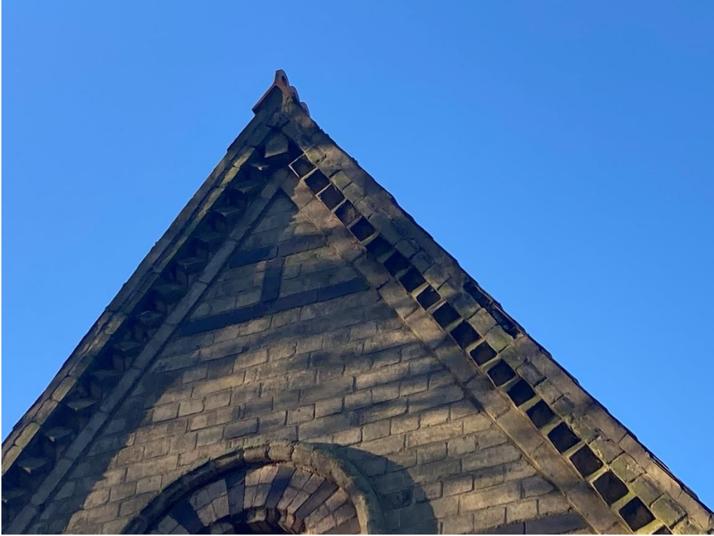
Missing or cracked verge pointing.
