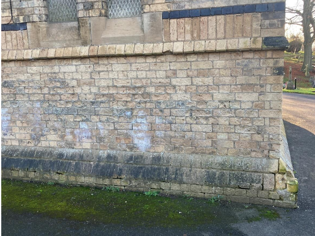
Band of cementitious mortar should be removed and repointed in lime.
