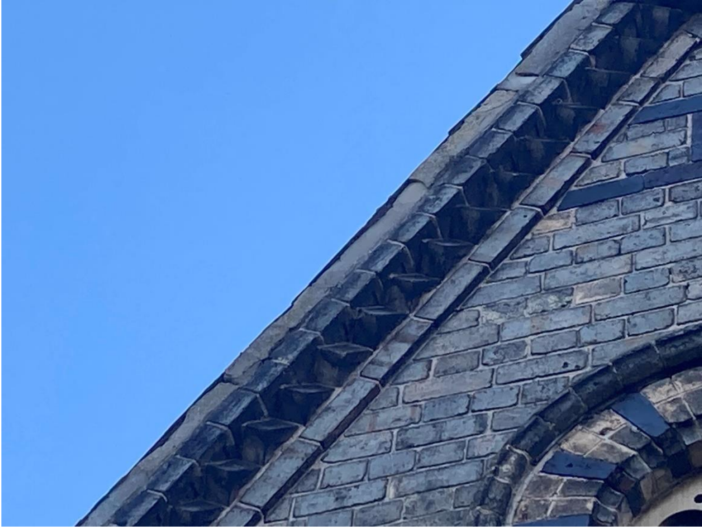
Missing verge pointing.
