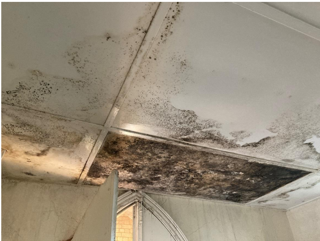
Heavy mould growth and water ingress to suspended ceiling.
