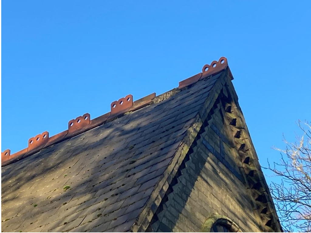
Missing decorative ridge tiles.
