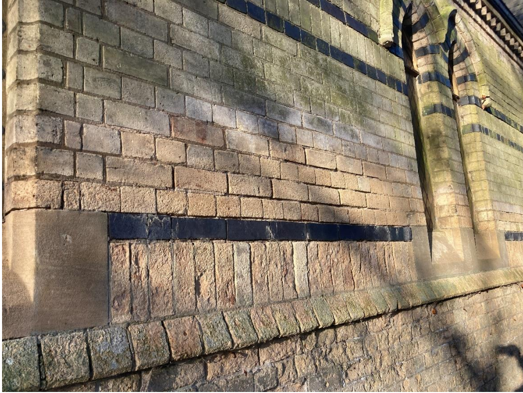
Open jointing to brickwork on East elevation.
