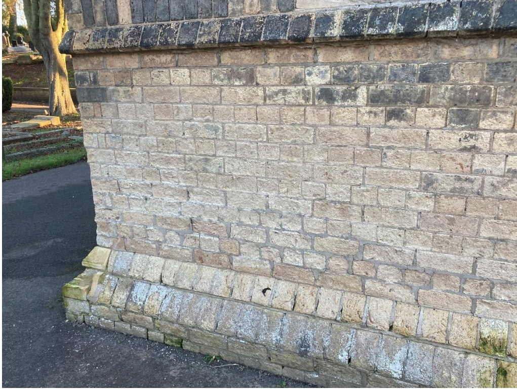
Cementitious pointing at low level should be removed and repointed.
